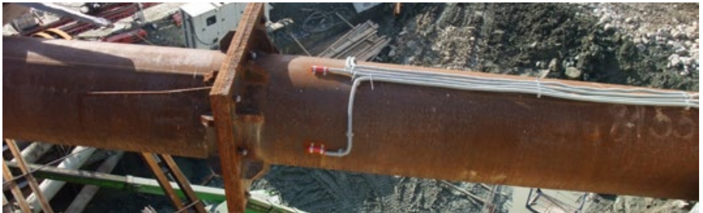
Spot weldable strain gauges on strut
